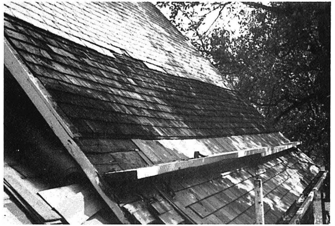
Removing slate and old wood shingles and installing new shingles 1663 House, South Side
