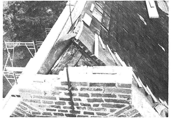
South Pinnacle Torn Down
